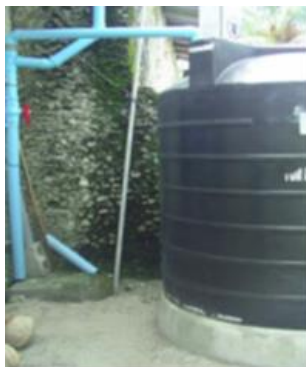
Figure 5: First Flush Diverter
